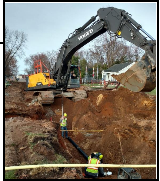
Smith St Water Main
